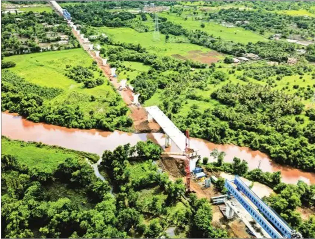
Construction of bridge over Darotha river is underway under Mumbai-Ahmedabad Bullet Train project, in Valsad, Gujarat
